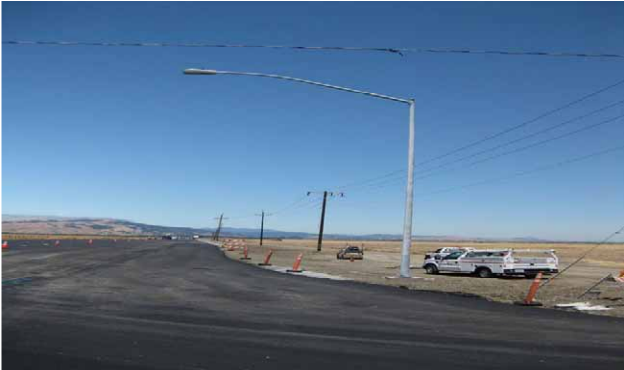
New Lighting at Shore Rd and Hwy 25
